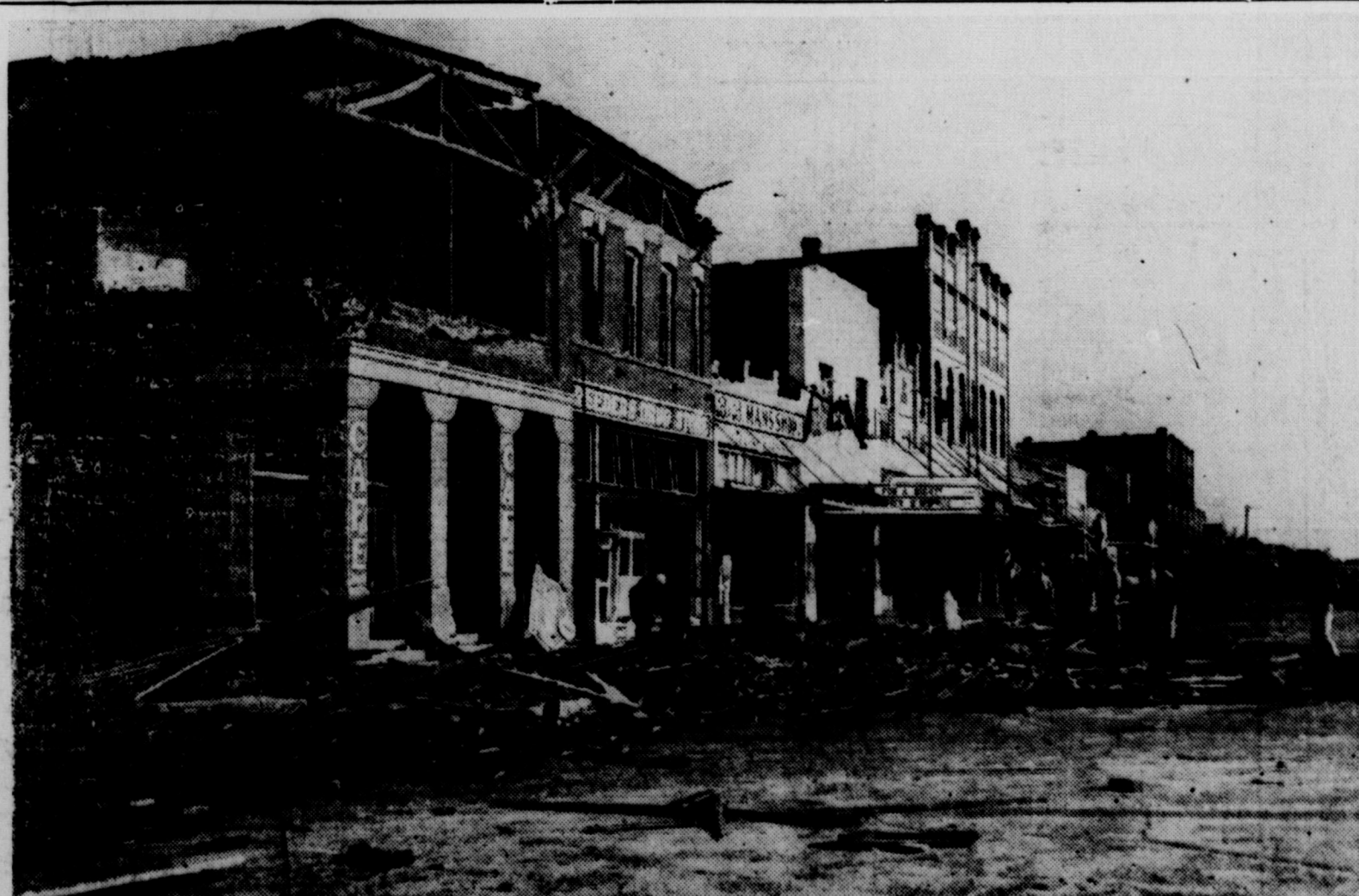
Looking north on the east side of the square at Crowell is the view of tornado damage. No business in this block escaped damage. Note that the highest structure, right center, whose front roof towered over the other buildings, was not damaged severely.
