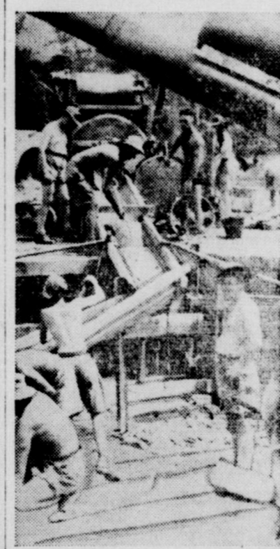
Australian soldiers are pictured concreting a gun emplacement near Darwin, in northern Australia, as they prepare to meet the onslaughts of the invading Japs. This is in the MacArthur theater of operations, where sizeable U. S. fighting forces have joined with their Anzac brothers. Note the colorful campaign hats.
