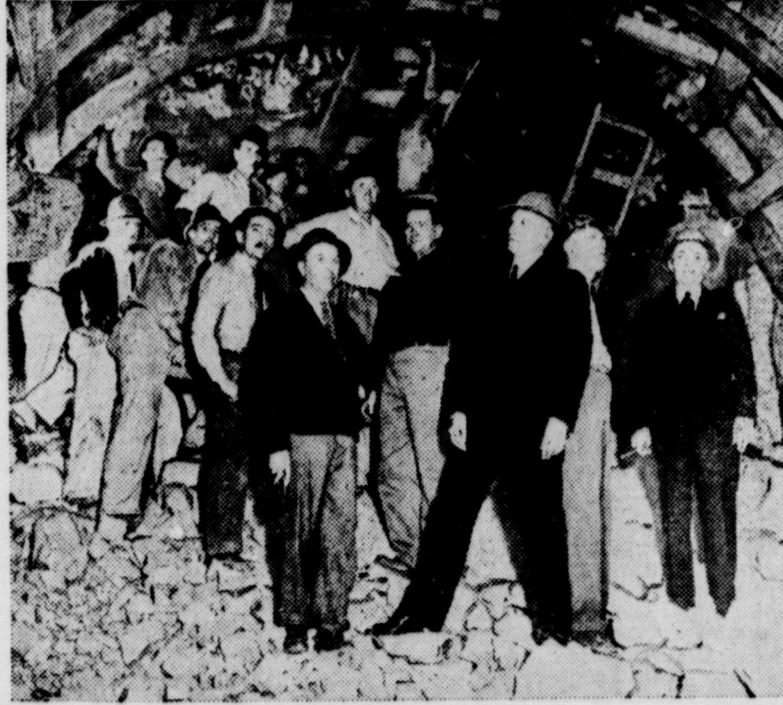
Interior of East Coachella tunnel in California, the longest tunnel in the world, after a charge of dynamite tore out the last barrier of rock and holed-through the 242-mile-long bore. The tunnel will carry water from the Colorado river to Los Angeles.
