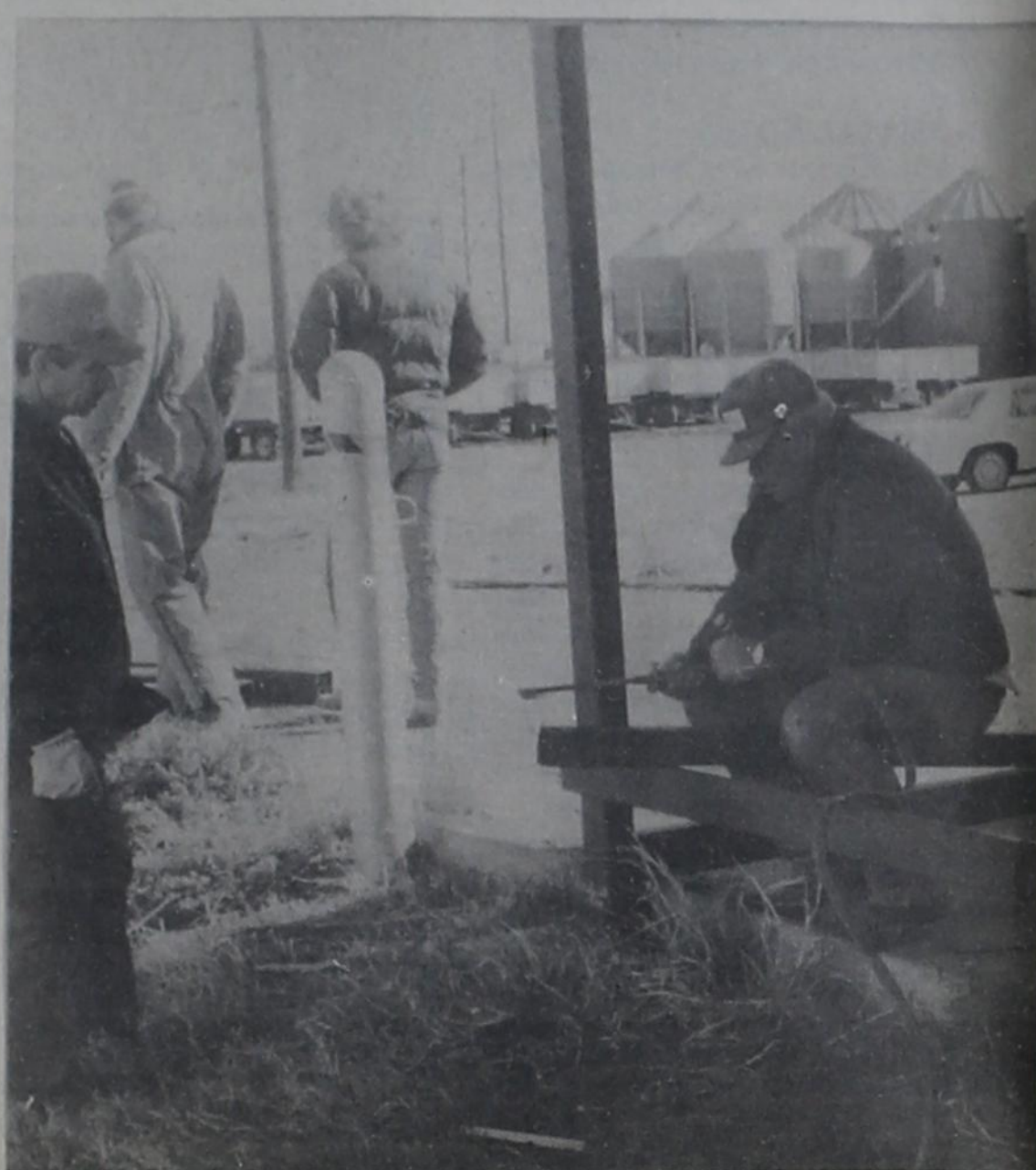
LLOYD WELCH busily works on the wash rack area of the newly remodeled building which will become the home of the Knox County Junior Livestock Show. Brazos Valley Young Farmers, sponsors of the county show and owners of the building, have made a number of improvements in the former potato shed in preparation for this weekend's show.
