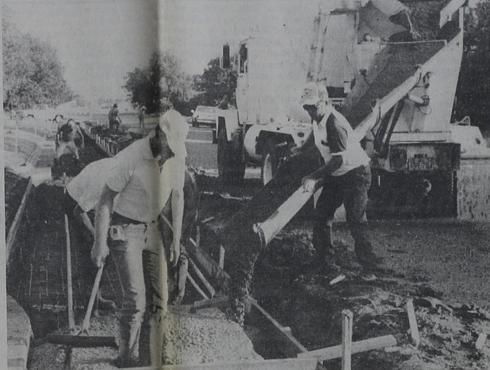
A PROJECT LONG-AWAITED by residents of the North Park addition in Munday is now underway. A drainage ditch is being dug along North Munday Avenue in hopes that it will alleviate the problem that occurs in this part of town after any large or heavy rain. John Lee Wilde, right, of the building company of the same name, directs the concrete into the ditch as an employee, Terry Bufkin, helps other workers to smooth the substance along the trough.
