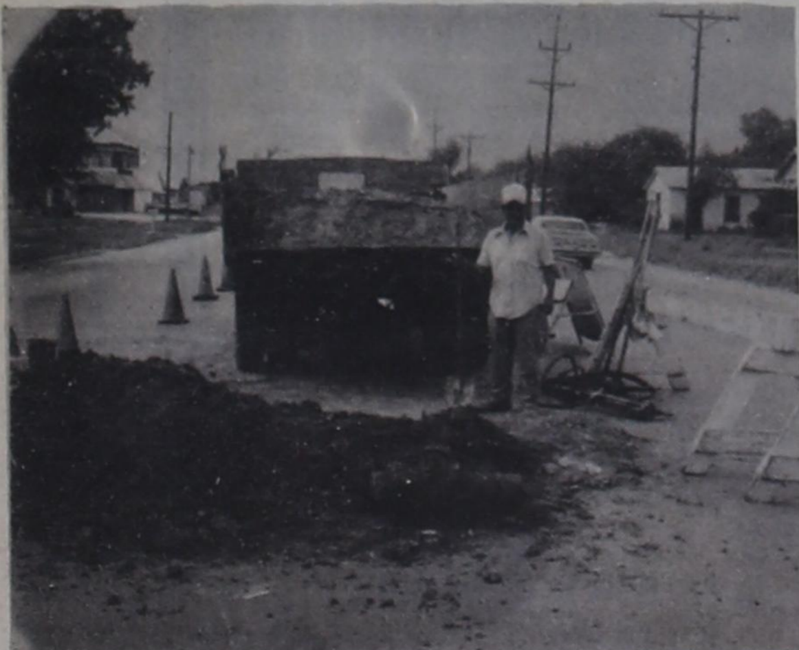
TAX DOLLARS AT WORK: City of Munday employees worked this week on another in a series of water line and cutoff valve repairs. Traffic was routed around the site on Highway 222 at the intersection of South 7th.
