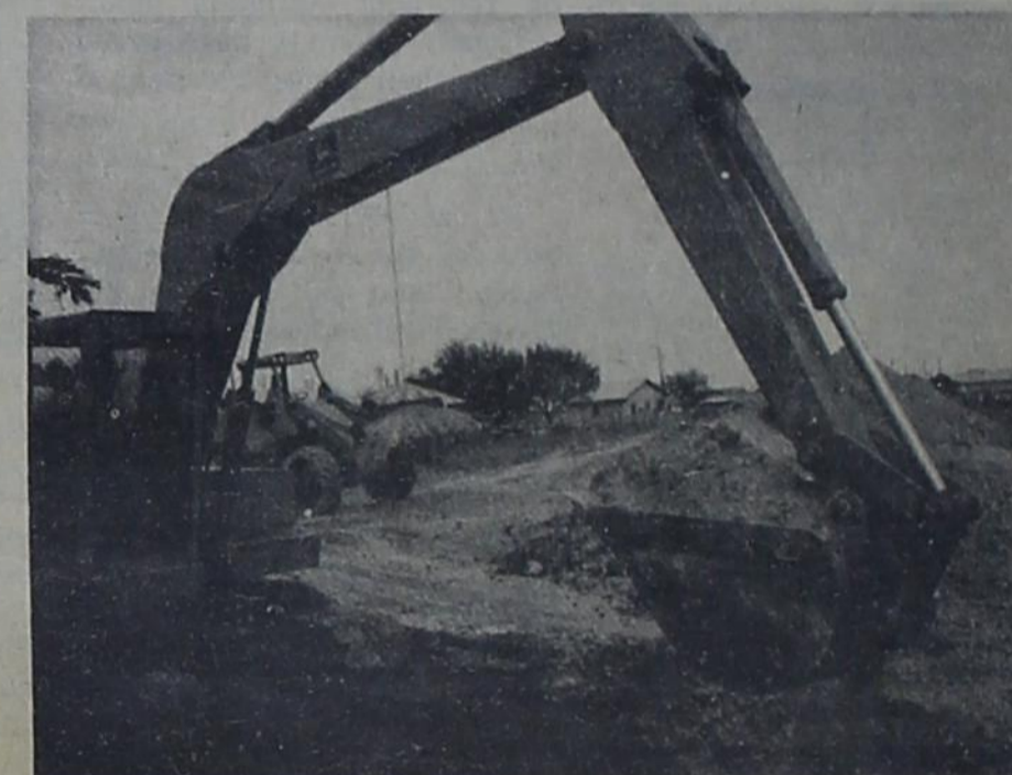
THE BACKHOE MACHINE shown here is digging the hole where the three pumps will be installed which will pump the water to the ditch.
