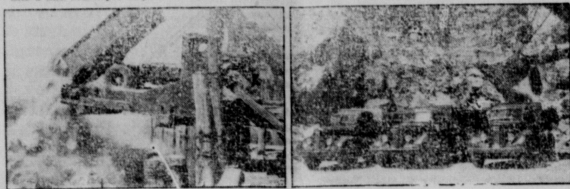
Half of the sea wall for the island was transported by CMC trucks from the quarry to sea-going barges that dropped the big boulders into place. Photos below show the trucks at work in the quarry and loading one of the huge barges.
