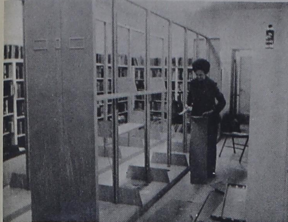
MRS. EDITH HOBERT, librarian, is shown working on the new shelves that had to be assembled. Donald Hobert and M. M. Booe were responsible for the major part of the frame work.
