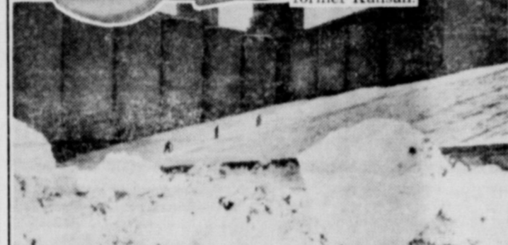
'ALPINE SCENE' in Kansas is actually view of rooftop of grain storage elevator, where workmen are clearing 19-inch snowfall that caused one section of roof to collapse.
