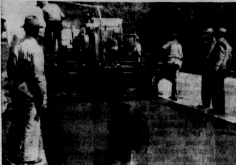
Laying a rubber road in Virginia. Particles of natural rubber are mixed with the asphalt surfacing to increase wear and reduce skidding.
