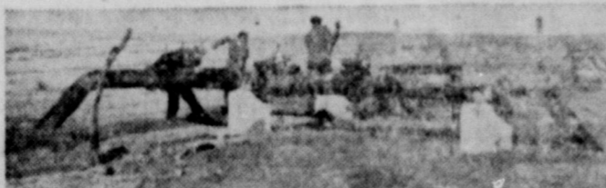
BEHIND GAS SERVICE there is something to build, paint, or repair every day, oftentimes in remote places. Above, a crew completes a control valve installation, part of a new compressor station. In the last three years, Lone Star has invested over $100 per customer to assure dependable service. Yet, you enjoy conveniences and comforts of natural gas service for a year around average of less than 15c a day.
