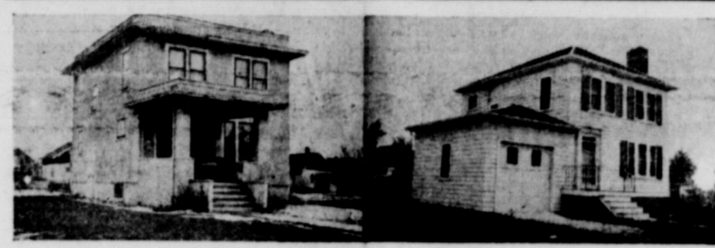
The possibilities that lie in modernization of old homes could hardly be illustrated more graphically than in these pictures of a Home Owners' Loan Corporation home. The cracked and discolored stucco was removed, and fresh new clapboard siding was substituted. The old-fashioned porch was trimmed down to 1940 proportions and a garage was attached to the house. A simple hip roof served to give new symmetry to the remodeled home. Private lending institutions make loans for this type of work, and these alterations are eligible for financing under the Modernization Credit Plan of the Federal Housing Administration. Even construction of the garage could be financed under the FHA plan, as it became a permanent part of the house.
