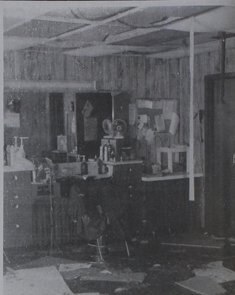
SHEAR LOOKS, owned by Diana Moore, was one of two local beauty shops that received considerable water damage when their ceilings fell through. Stacia's Coiffures , just a half block down the road, was the other one, owned by Stacia Cook.
