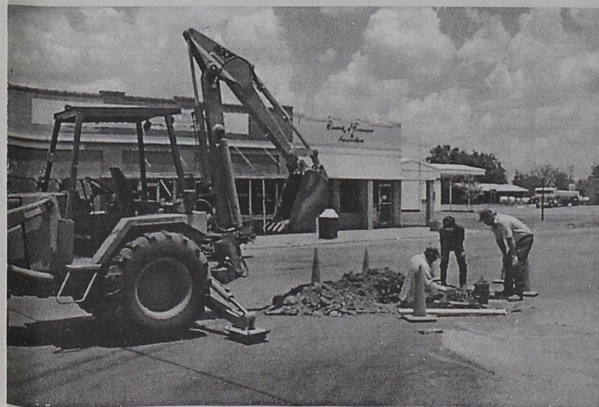
CITY EMPLOYEES worked in the hot summer sun over the week-end and into the first part of the week to fix a leak that developed in the water lines. Regardless of the temperature, work goes on across the city.
