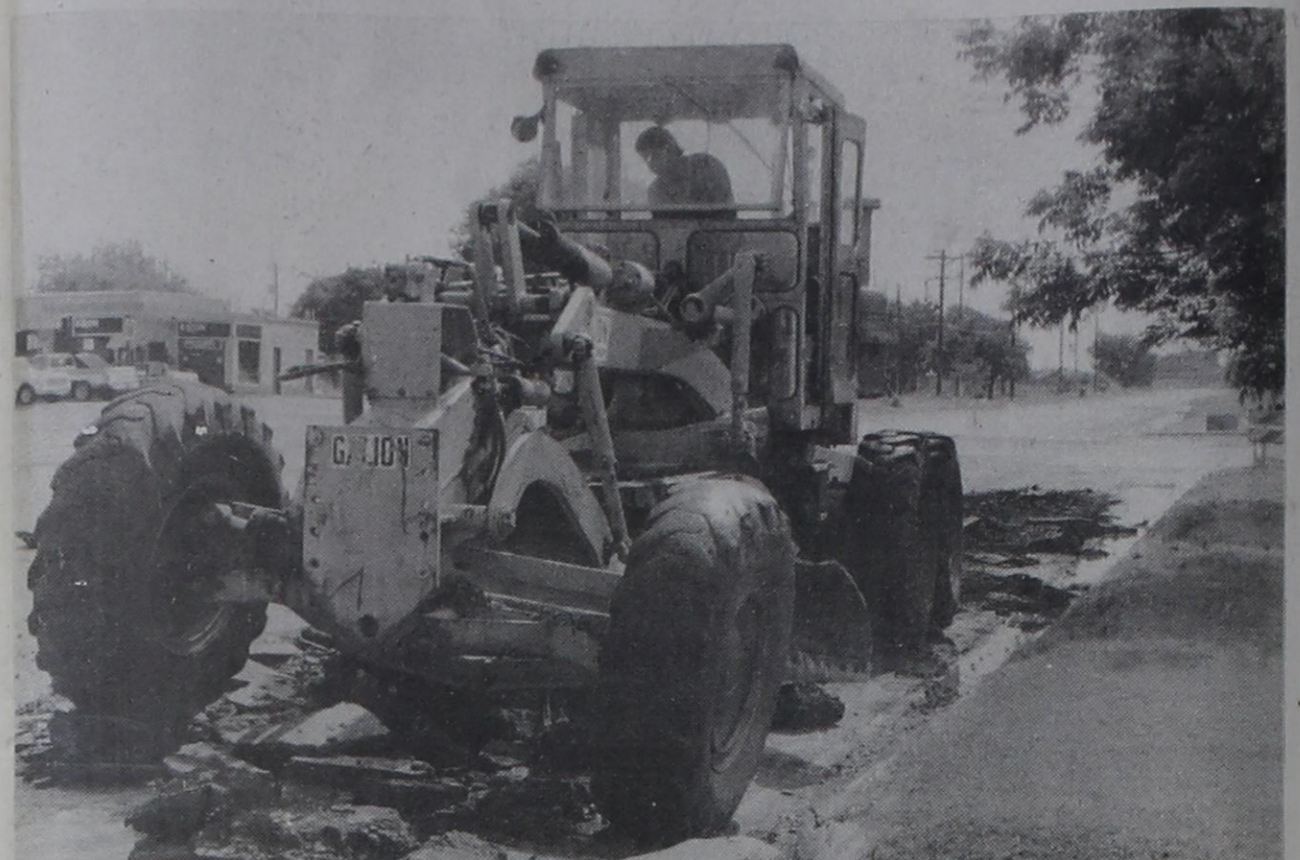
IN CASE YOU HAVEN'T NOTICED . . . the road in front of The Munday Courier is a mess!!! The city crew started tearing up the road over a week ago, one day before all the rains came. That stopped them from doing any further work. Please bear with us a while. It should be a big improvement when the job is finally finished.
