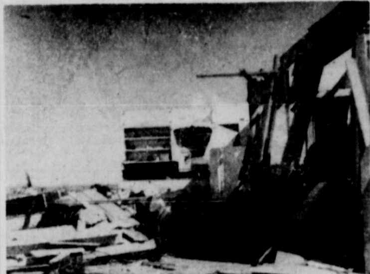
ONE DIED HERE — This is the living room of the W. W. Hyde home. The chair in which he sat drinking coffee when the storm struck is behind collapsed door at right. His body was found in the debris strewn here.
