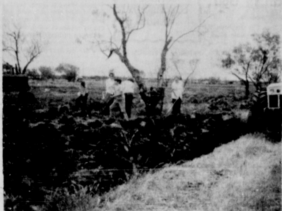
WORKERS WERE 'HARD AT IT' when this photo was taken as they began clearing the ground Saturday for the Benjamin Park. The workday had been postponed twice previously but Saturday's weather was ideal. [Benjamin Photo]
