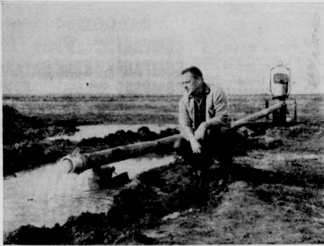
GOOD WELL — Sonnie Hughes, owner of Irrigation Products Company, is shown beside the well he dug last Tuesday. The City Council met to discuss the purchasing of the well, but hadn't reached a decision by press time late Wednesday. The well is pumping approximately a five and one-half inch stream and is located just south of the city limits of Knox City.
