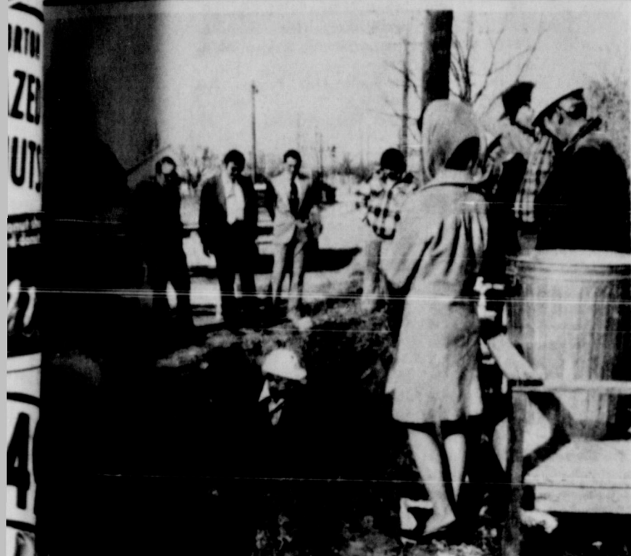
REPRESENTATIVES FROM LONE STAR GAS CO., the Texas Railroad Commission, and the City Council were on hand Monday afternoon to observe the installation of the gas company's underground pipe. As Gerald Stephenson, inspector of Dallas inspects the pipe, those observing include, reading from left, Mayor Kenneth Crowover, Joe N. Brown, Norman Langham, M.R. Lester Yates, Eddie Wright, A.T. Holcomb, A.P. Denton, Charles G. and city secretary Faye Railsback.
