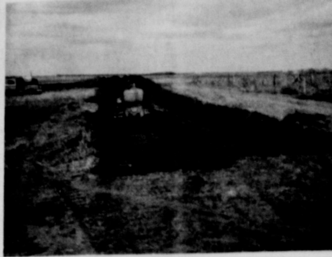
CITY'S NEW DUMP GROUND — Work began Tuesday of this week on dump ground facilities for the City of Knox City. Jay Eaton, Caterpillar operator is shown above as he began digging on city property north of the sewerage disposal. Officials have tried unsuccessfully for the past two years to obtain more land for dumping purposes. Decision was made to use the two acres already owned by the City and to make the grounds accessible to residents, in the near future.
