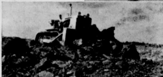
BEAR for work is this new International TD-25 crawler tractor, here moving huge load of earth on runway extension project at Chicago's jet-age O'Hare International airport.
