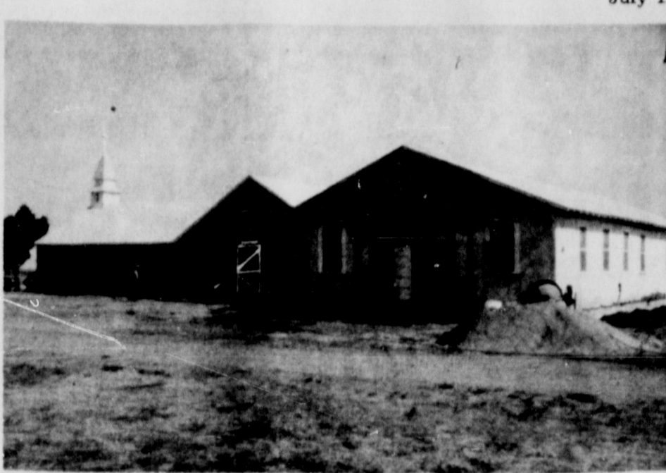
A NEW FELLOWSHIP HALL that will also provide several Sunday School classrooms has been moved behind the Gillespie Baptist Church and is presently being remodeled. A hallway will connect the two buildings, according to Ray Milhoan, pastor.
