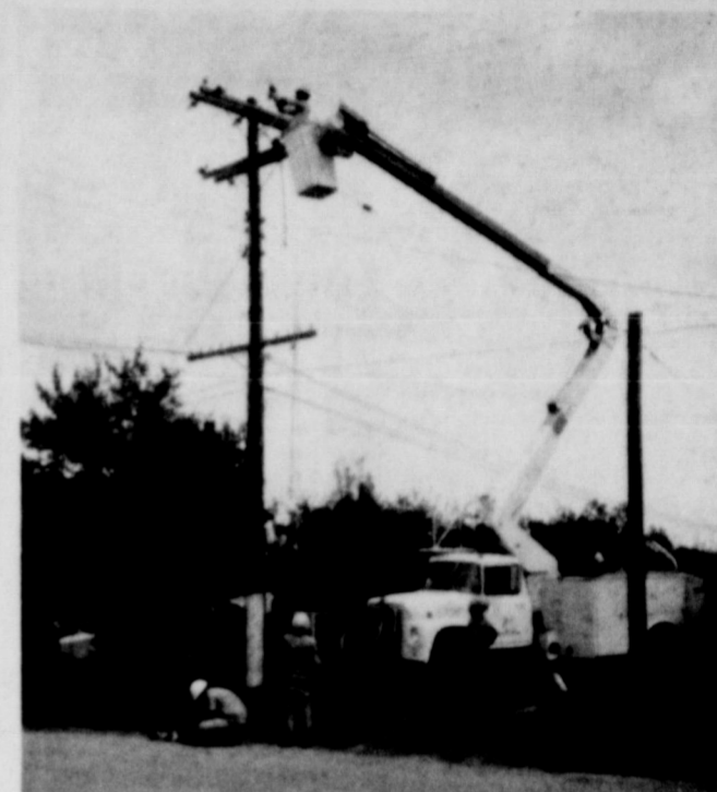
SHOWN HIGH ABOVE the ground in the bucket lift of the Pitman Hot Stik truck is Al Lewis working with insulated rubber gloves and handling hot lines of 4,000, 7,200, and 12,500 volts. Switching hot lines, townspeople were without electric service only about thirty minutes at a time whereas the current would have been off all day otherwise. George Field is shown near the truck and two out-of-town employees are pictured at left.
