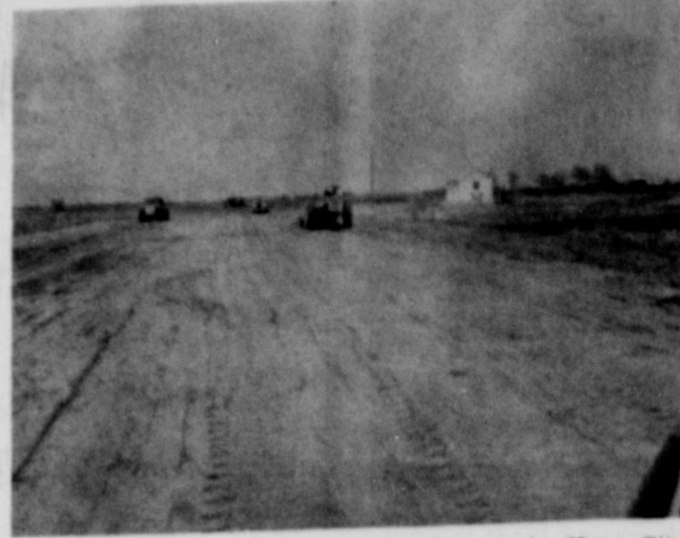
CONSTRUCTION OFFICIALLY BEGINS on the Knox City Municipal Airport. Heavy equipment is shown above, looking north, on the site of the new landing strip.
