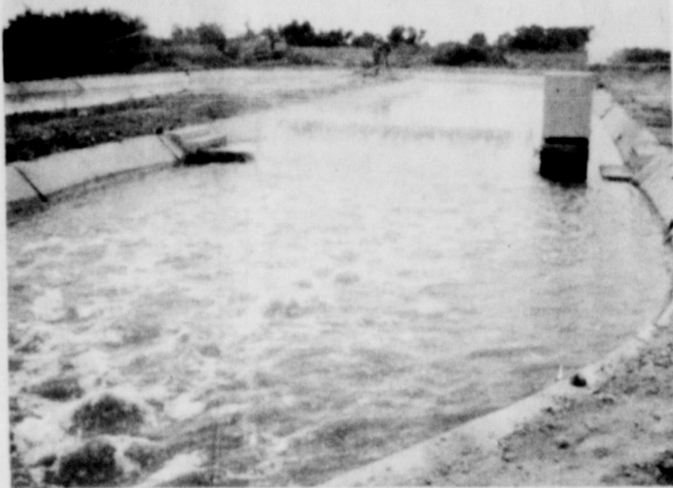
WATER WAS TURNED INTO THE NEW WASTEWATER TREATMENT PLANT northwest of Knox City Thursday of last week. The photo shows the concrete lined aeration ditch with the cage rotor that will operate continuously. A laboratory building has been installed on the site and is equipped with laboratory equipment as directed by the Texas Water Quality Board and the Texas Department of Health.
