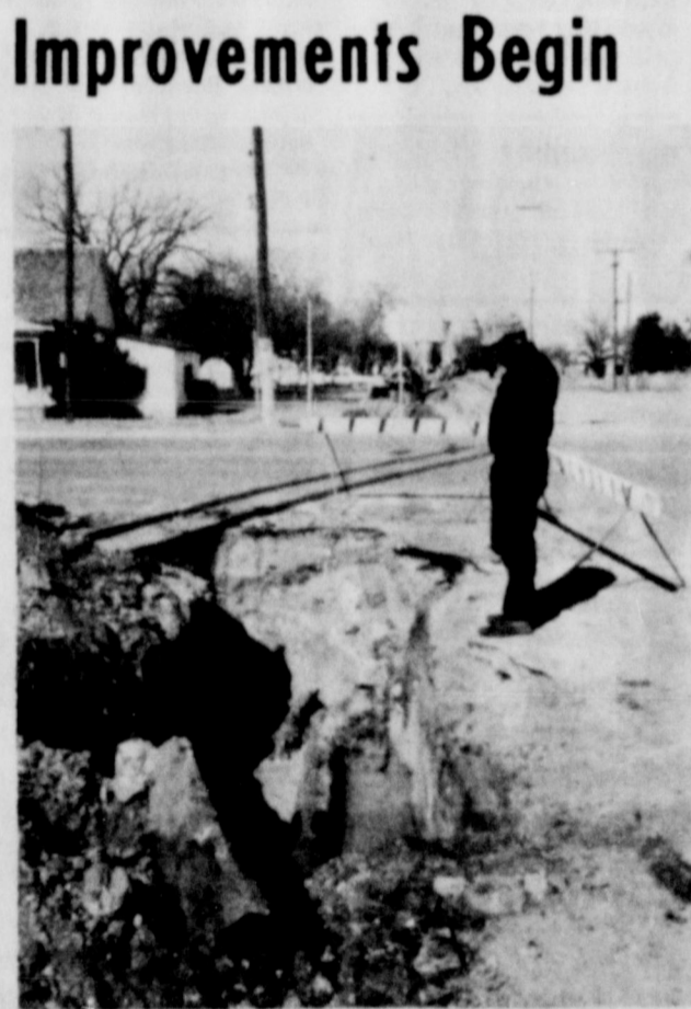
GOING UNDER STATE HIGHWAY 222 near the Conoco Station is this casing Bowles Construction Company of Burkburnett has begun laying to update the water lines in Knox City. Jimmy Garcia of Wichita Falls, pictured here, is supervisor for Bowles.
