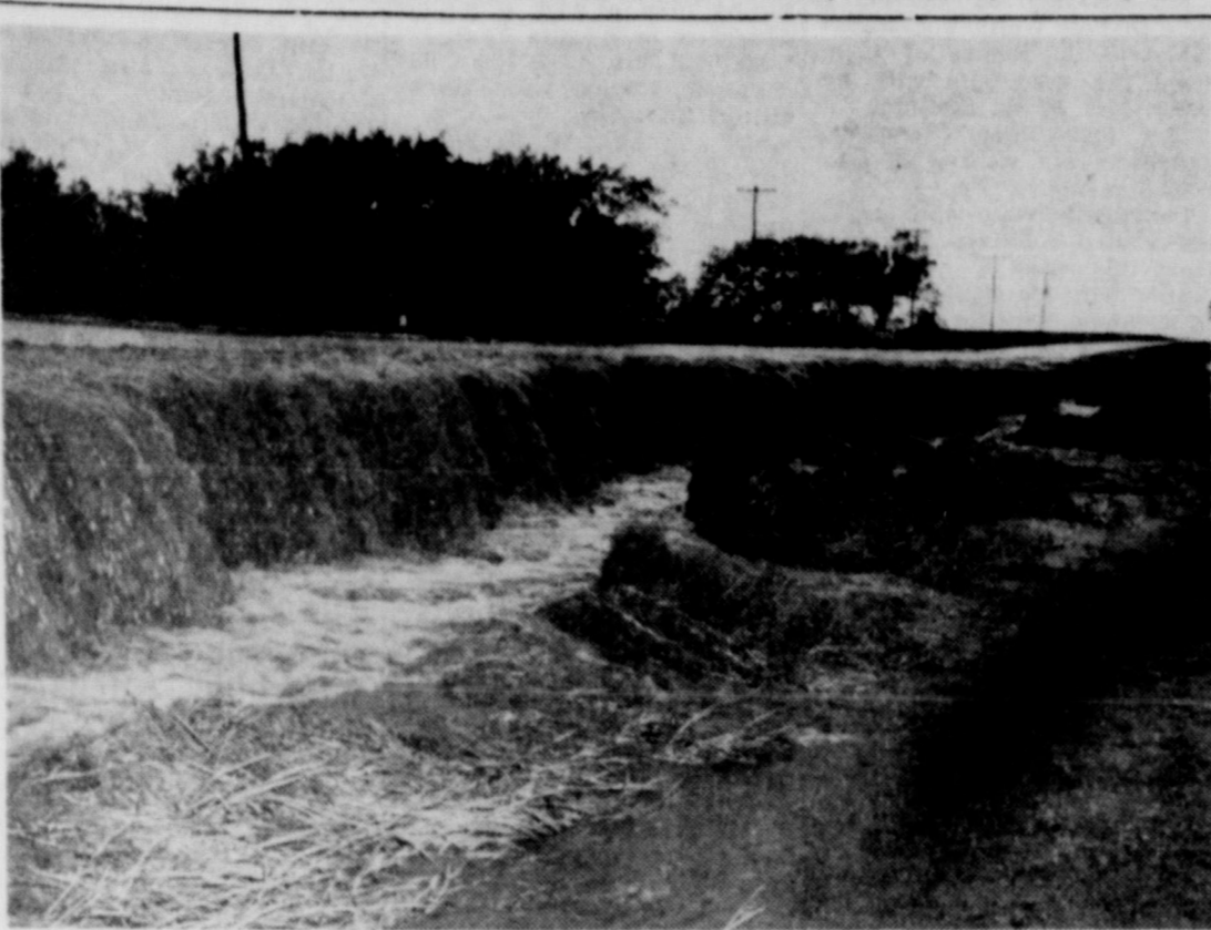
No, this isn't Niagara Falls, but it looked like it Saturday when the rains ran "China Draw", just over the pavement. The deluge cut away the shoulder of the road and endangered the pavement and the concrete culvert before the water receded.
