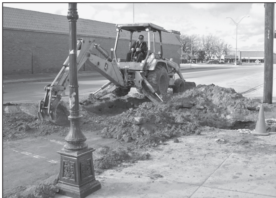
FINISHING TOUCHES —Tony Williams puts the finishing touches on this water main repair that occurred during the recent cold spell. City Administrator Brandon Anderson reports that during the cold spell the city had a total of nine breaks. A few more small leaks may surface yet. The City feels fortunate that only a few leaks occurred as this was some of the coldest weather that Haskell has experienced in quite some time. Mayor Bob Smith and Anderson would like to thank the City's Public Works employees who had to work overtime in these cold conditions to help keep our customers supplied with water. The City of Haskell would also like to apologize for any inconveniences these leaks may have caused our citizens.
