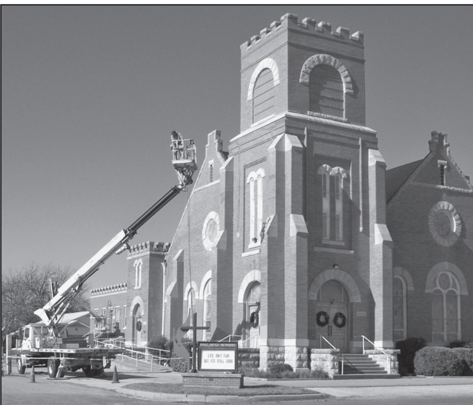
CHURCH WORK —This sky high crew is doing tuck-point work for the First United Methodist Church in Haskell. The project should continue this week.
