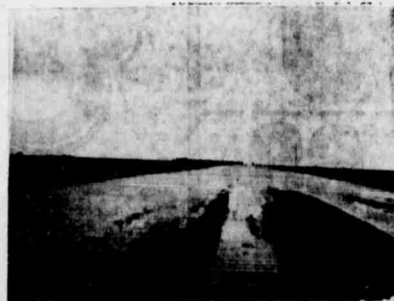
This picture shows one of Haskell County FM Roads heavily inundated by runoff water due to lack of sufficient water control on the watershed above the FM Road.
