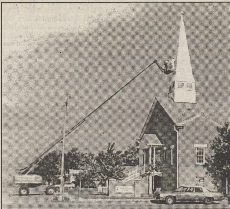
Painters have been using this unique ladder to paint the steeple and cross on the Silverton United Methodist Church. Windows in the church also are being replaced. At least one church member dared to venture up the ladder to have a look "from way up high."
