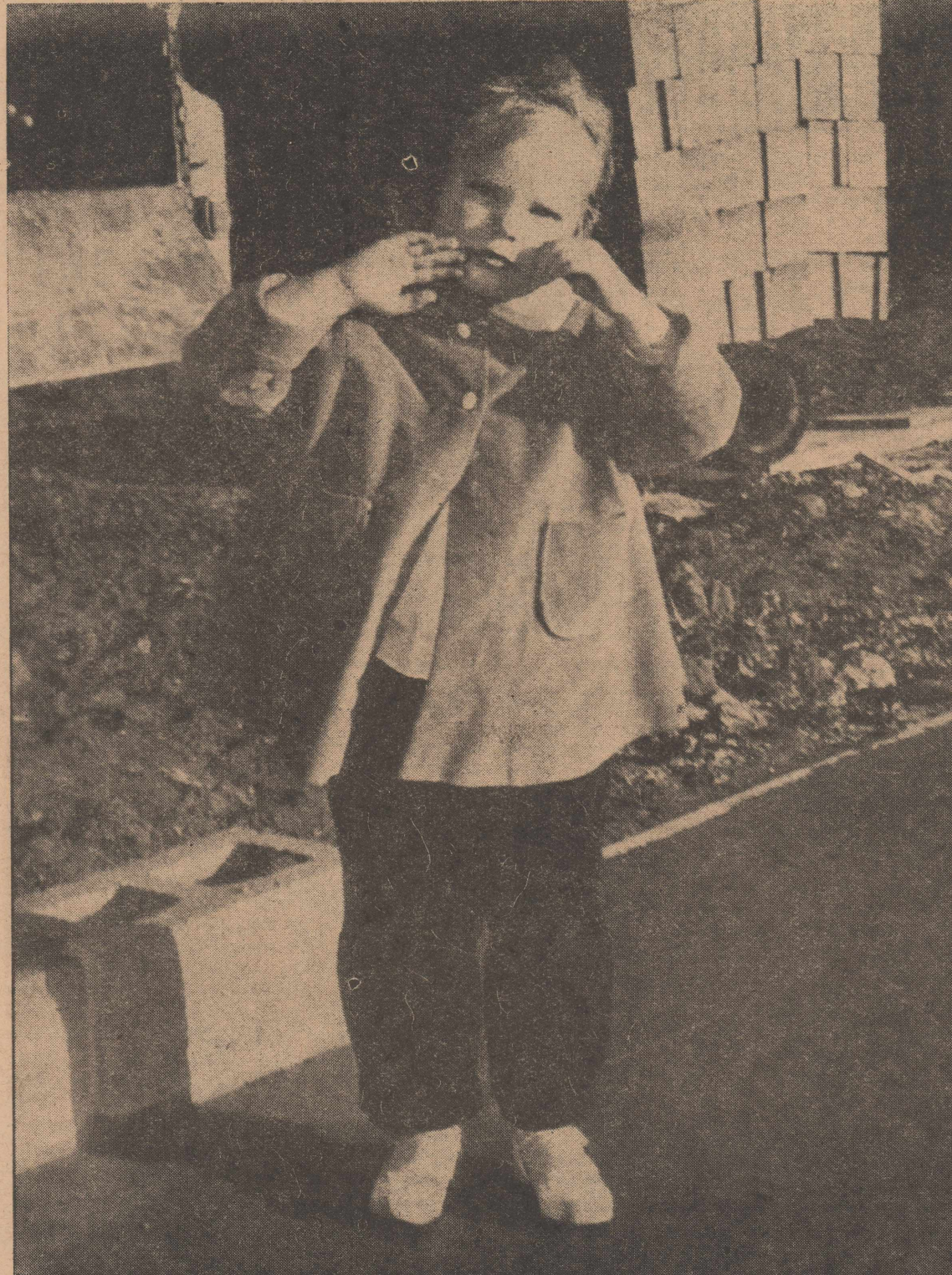
Kaysee Martin, 3-year-old daughter of Publishers Troy and Korkye Martin, stoically braved wind and sand Tuesday afternoon to put her footprint in the new concrete of the floor of the new Olton Enterprise Building. Plumbing is complete on the new building and masonry work is to begin as soon as weather permits. (STAFF PHOTO)
