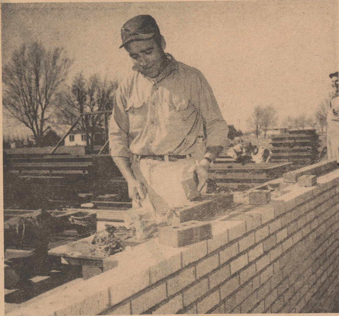
Putting the brick on Olton's new elementary building is Leo Tech, bricklayer from Littlefield. He is a member of Local 23 of Lubbock and has been laying brick since 1946. Work is progressing smoothly on the new building. (STAFF PHOTO)
