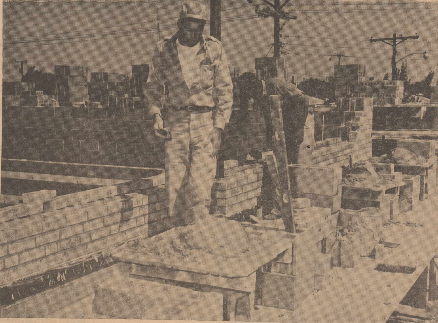
Work appears to be progressing on schedule on Olton's half-million dollar school plant improvement. Workmen are shown here laying bricks for the fine new gymnasium. (STAFF PHOTO)
