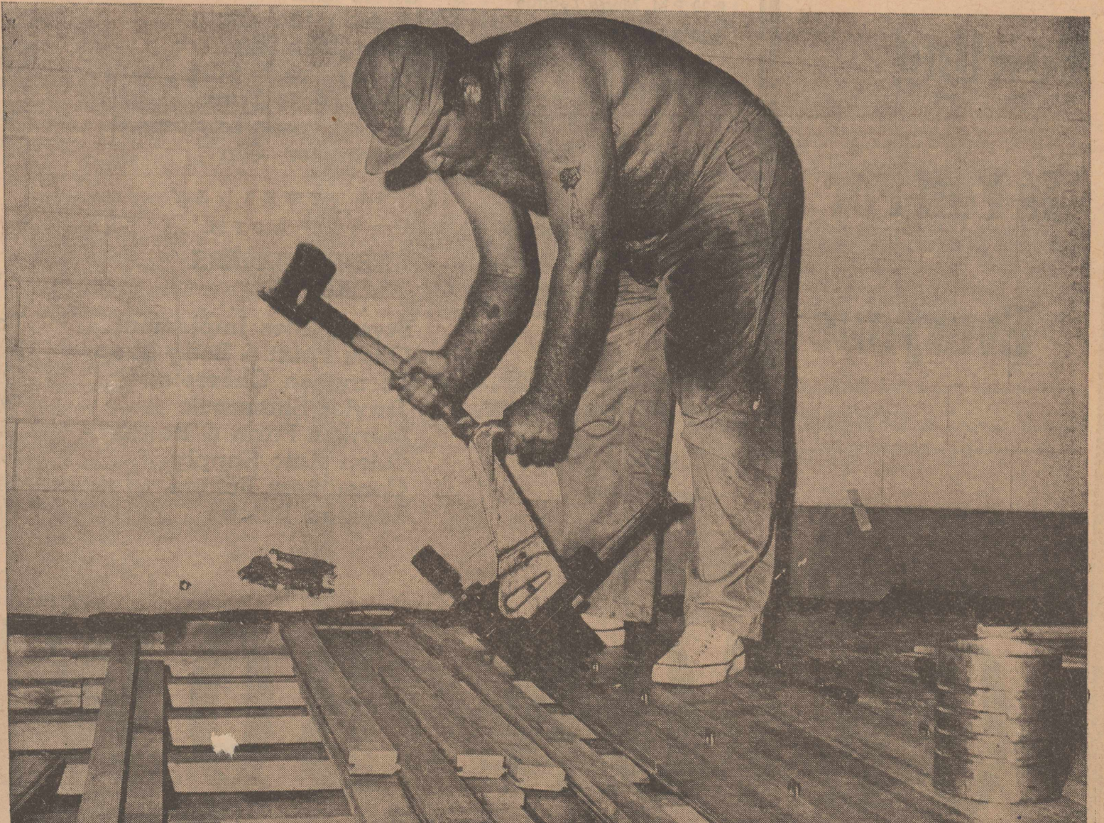
Olton will have the first free floating gym floor in West Texas. The spacious new gym is scheduled for delivery some time in October. The resilient floor is credited with preventing injuries to athletes who use it. The floor is attached to wood slabs which, in turn, rest on porous rubber pads, giving the resilient effect. (STAFF PHOTO)
