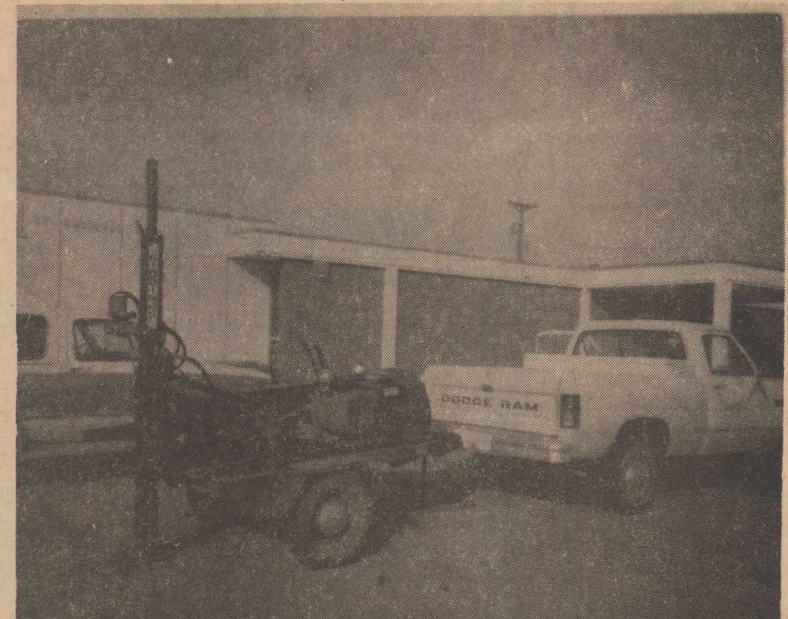
Core Drilling Unit Used By SCS Technicians Locating Pipe Location For Sub-Surface Drains.
