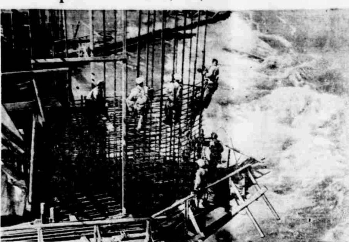
Army engineers are speeding the construction of the $32,400,000 Bonneville dam in the state of Washington. This interesting picture in which sky, water and steel meet shows workers erecting piers that will span the Bonneville river. This PWA project is a huge power, navigation and flood-control undertaking.
