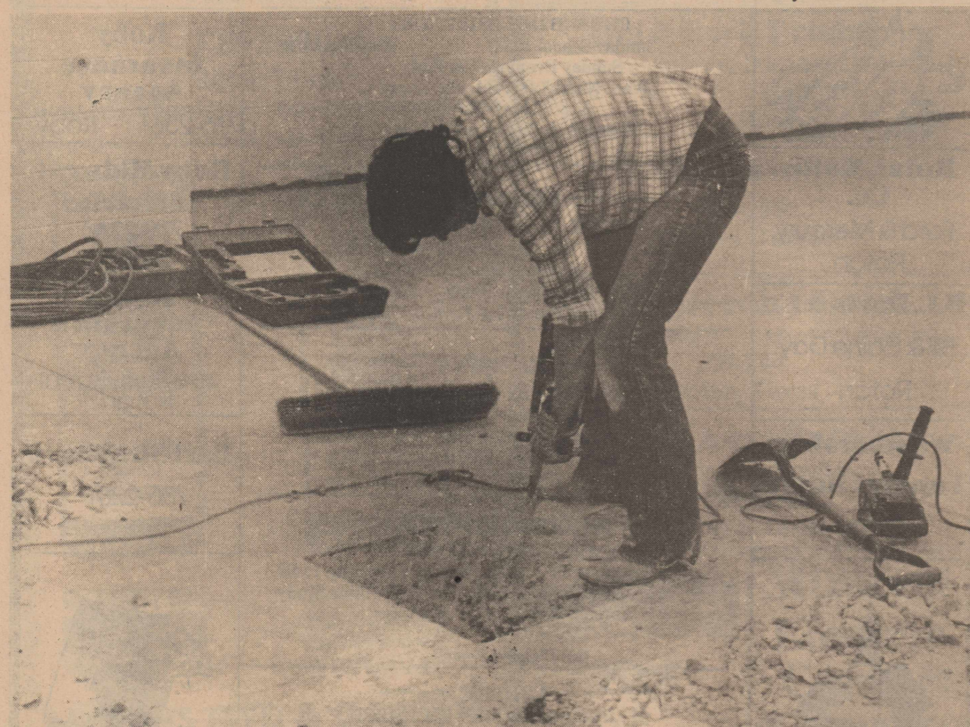
DRILLING THROUGH CEMENT: A workman drills through the cement floor of the new Roby gymnasium in preparation for installing volleyball bases. The new gym
