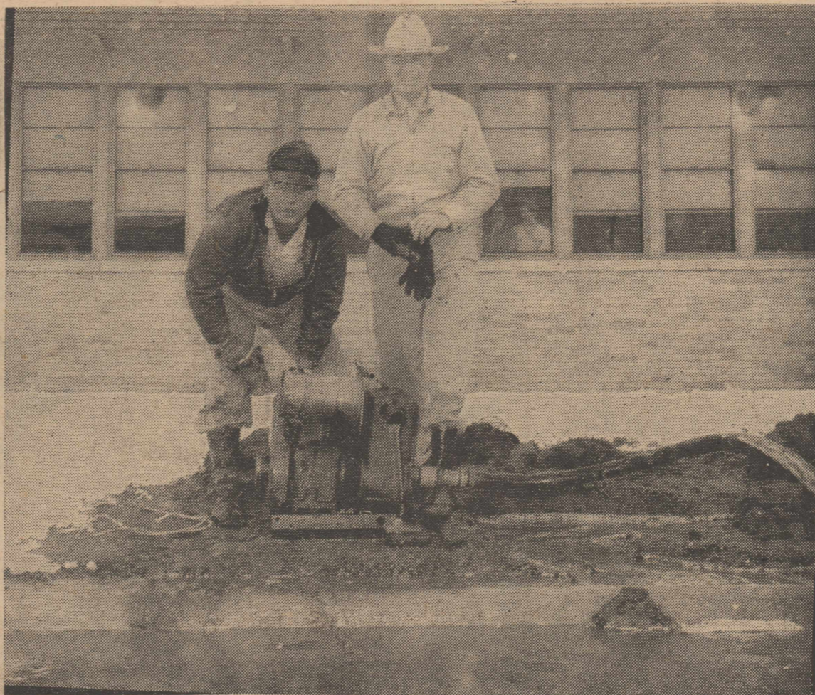
JEFF MARSHALL, left, city employee, and D. Y. Ray, mayor, were repairing a broken water line during last week's snow. The wet and cold work was taking place near the school. Their efforts didn't go unnoticed. The two girls who may be seen in the window behind Mr. Ray's left elbow served as an audience during the undesirable chore.
