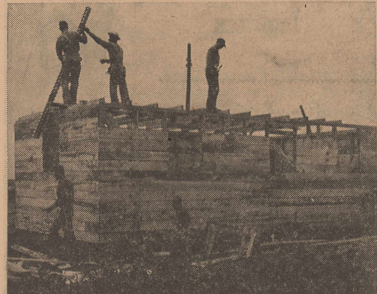
FIRST HOUSE goes up in reconstruction operations in South Olton. The city council is busy trying to improve the slum conditions which existed in this section before it was struck by the recent tornado here. (Staff Photo)
