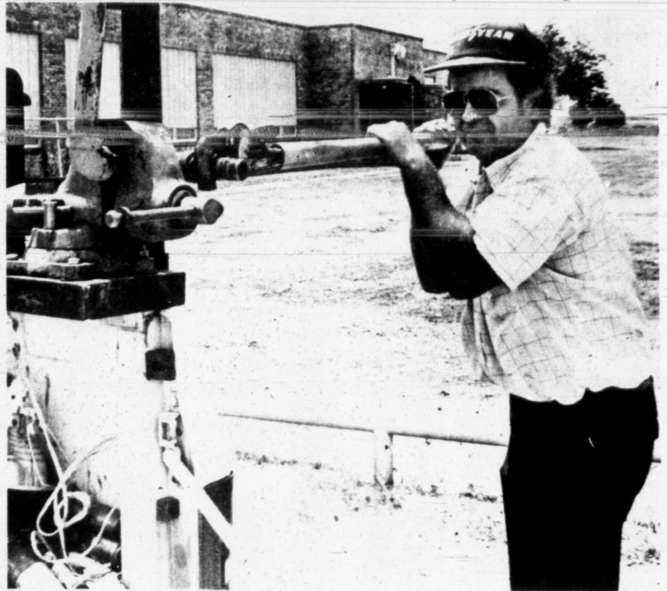
PIPEFITTER — Jesse Faulkenbery was putting pipes together at North Elementary School for the school's boiler replacement project. (SDN Staff Photo)
