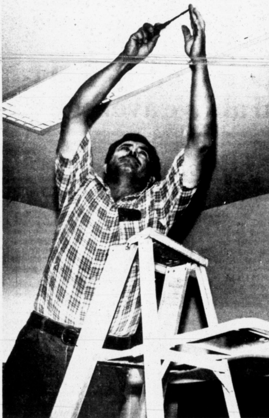
LIGHTS — Rudy Rodriguez was replacing fluorescent lights at Snyder Junior High School as maintenance men throughout the school district moved from school to school to get the buildings ready for a new population of students. (SDN Staff Photo)
