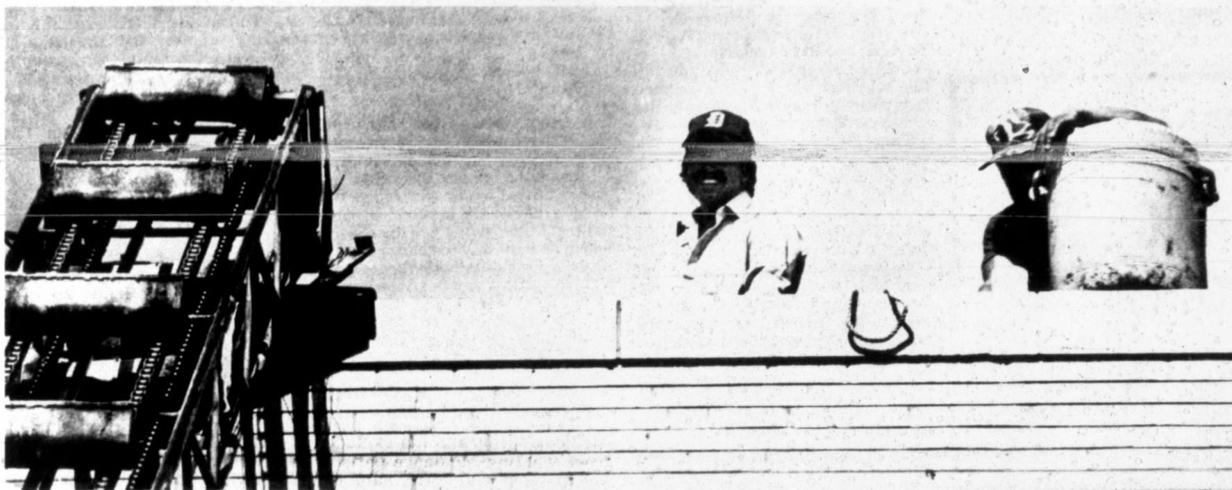
IT'S NOT TOO HOT TO SMILE — These workmen were putting down hot tar in 100-degree heat on the Snyder High School roof last week but were not too hot to show their amusement at finding themselves in a picture. (SDN Staff Photo)
