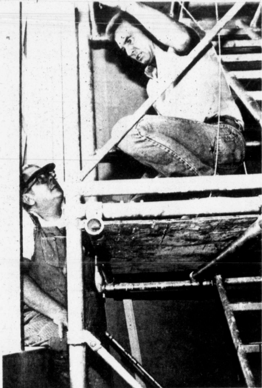
WINDOW-FIXERS—Bob Payne, left, and B. W. Harris were repairing windows last week at Snyder High School as the new school year approached. (SDN Staff Photo)
