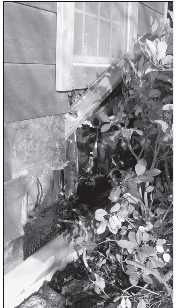
HOUSE FIRE —Minimal damage was sustained Thursday afternoon, Jan. 22 to the home of Mark Wallace located on S. Third East in Haskell. A family member had returned home to find flames coming from below this southern-facing kitchen window. The interior of the home suffered little fire damage, but smoke filled most of the home. The cause of the fire is under investigation.
