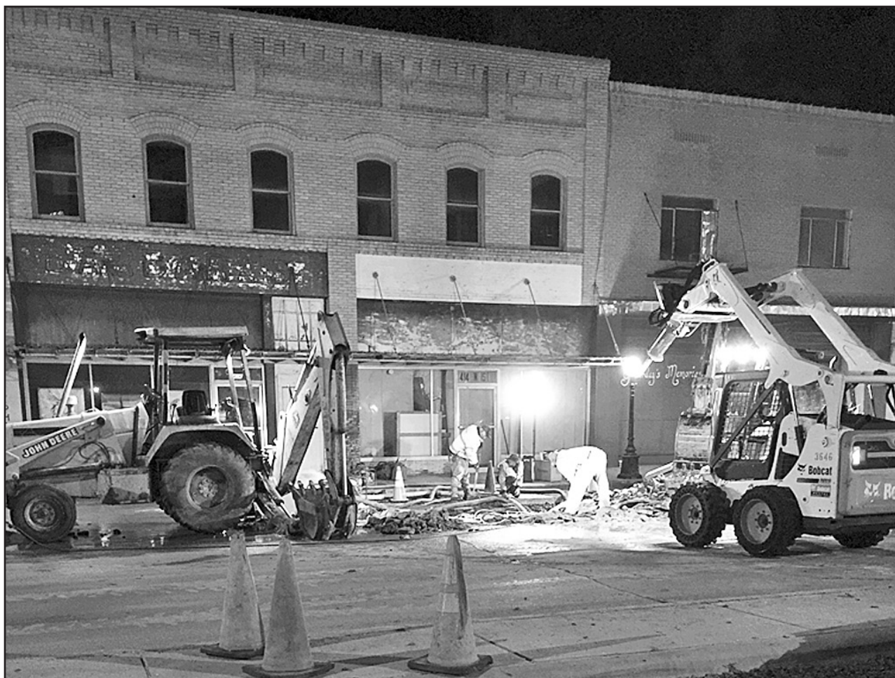
WATER LEAK —City crews had a large water leak to repair on the north side of the square Saturday evening, Jan. 2. The break in the 8 inch main line was due to the aging infrastructure and stresses of weather. The City wishes to thank the Haskell Volunteer Fire Department for their help, and the citizens for being understanding during these unpredictable events.
