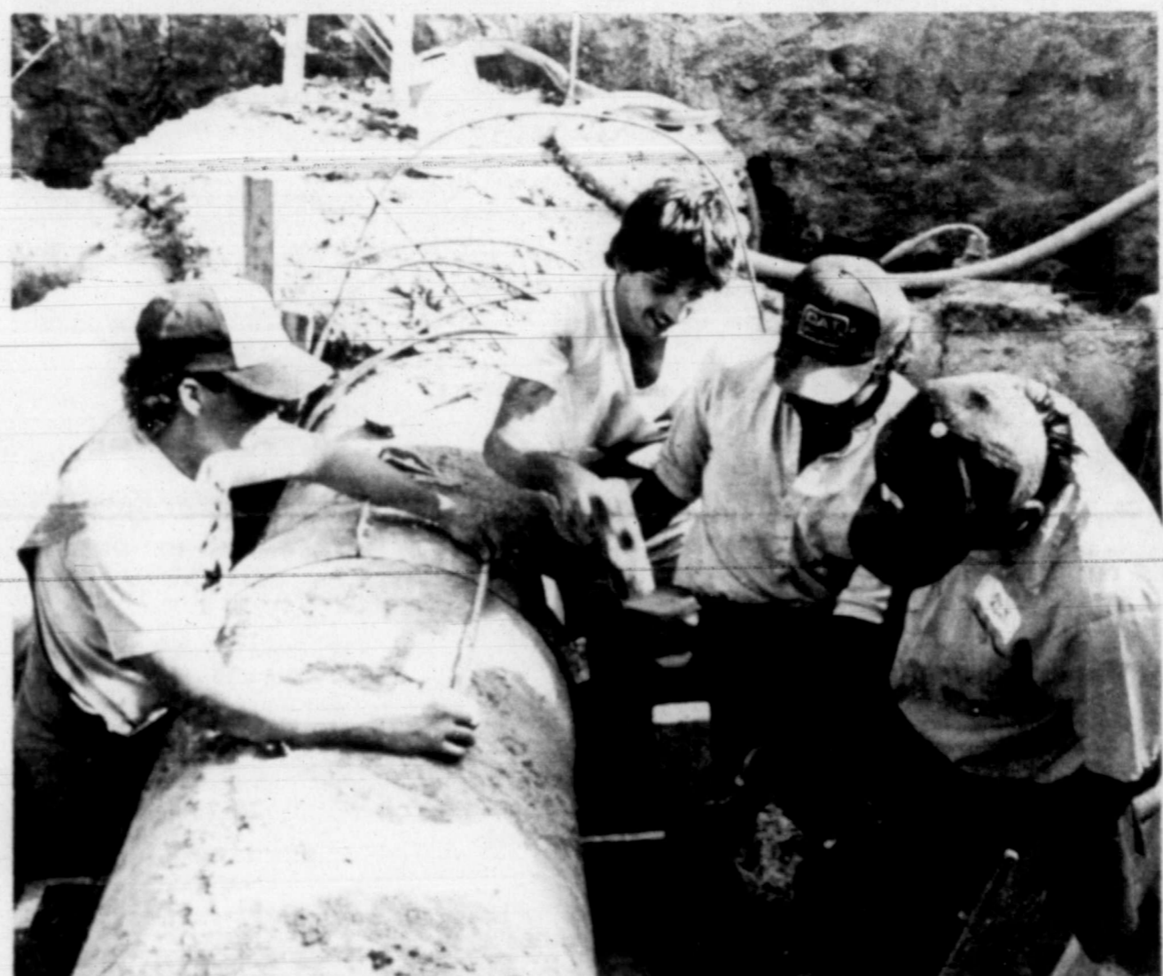
HAMMER DOWN — A construction crew works on the follow-up of connecting a looped 24-inch water line from the new rapid mix basin at the Ave. M water treatment plant to the Lake J.B. Thomas line Thursday afternoon. The connection was made Thursday morning. It followed a 20-hour plus period during which the city was dependent on its stored reserves. (SDN Staff Photo)
