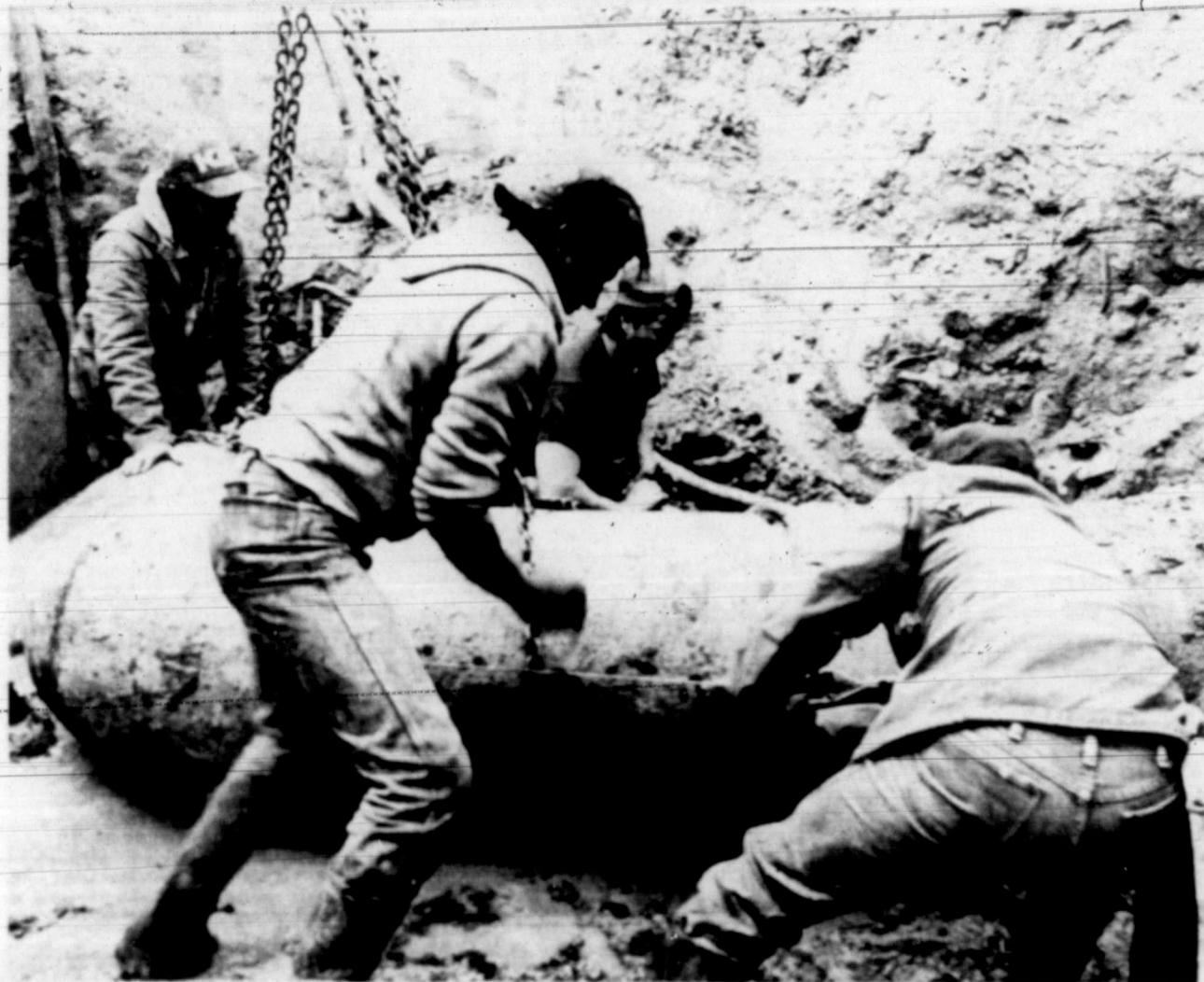
MAKING THE CONNECTION — After several hours of work, a Decker Construction Co. crew from Abilene pushes home one end of the 24-inch L-shaped pipe connection which fits a new rapid mix basin at the water treatment plant to the main line from Lake J.B. Thomas. The city's water supply
