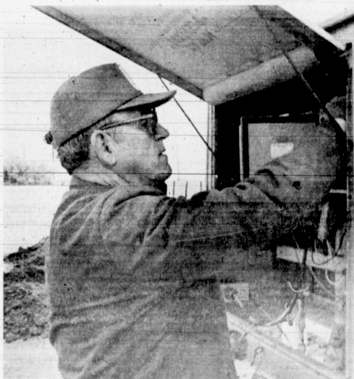
COLD WORK — Long Star Gas Co. service specialist Cliff Necessary works to keep the line pressure up manually at the W. 37th St. Lone Star station Thursday morning while equipment was being repaired to keep the pressure up
