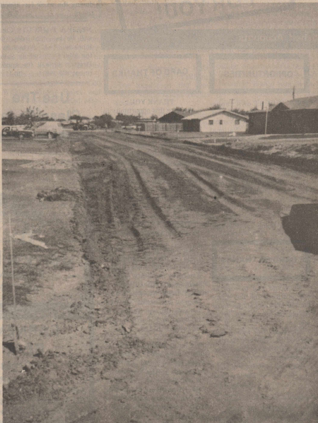
THE MUCH NEEDED RAIN has slowed down the long-awaited paving project on Aspen Street, but the preliminary work has begun. Lipham Construction Company of Aspermont is contractor.
