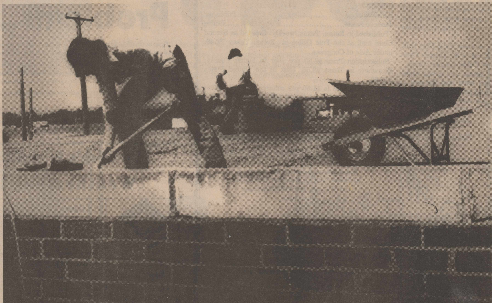
FIXING ROOF: Workers of the Herb Stevens Roofing and Insulation Company of Plainview began work to install a new $75,000.00 roof on the Rotan High School and Elementary School last Monday. Rotan School
