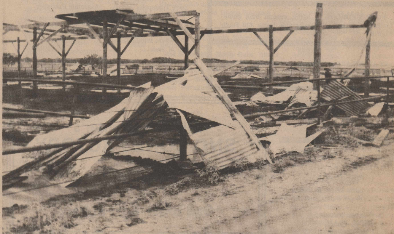
A TORNADO did extensive damage last Thursday afternoon at Brazos Valley Feeders northwest of Rule. Three sheds had the roofs torn off and dumped, steel pipe fences were ripped apart and twisted, and three head of cattle died in the storm. (News Photo)
